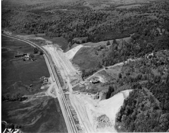
Oblique aerial photograph shows construction (excavation and blasting) of Interstate 89 in Montpelier. Note cleared land at left, most likely farmland. Uplands are densely forested. Route 2 and train tracks are visible. LS06207
